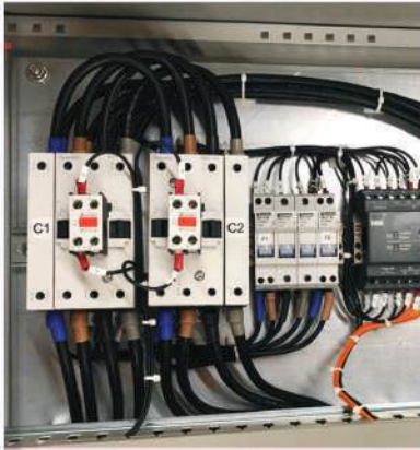
Auto Transfer Switch (ATS)
