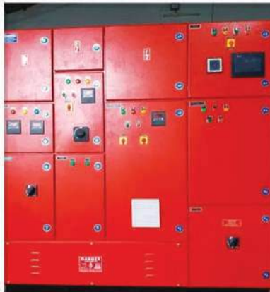
Fire Fighting Panels
