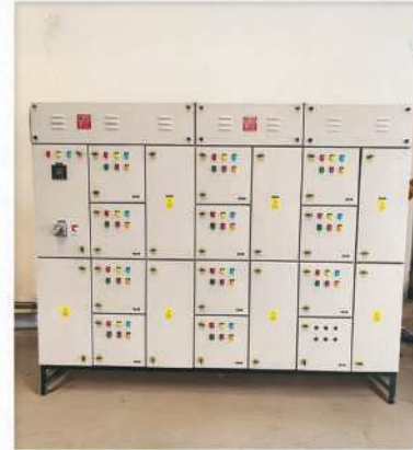
Motor Control Center (MCC)
