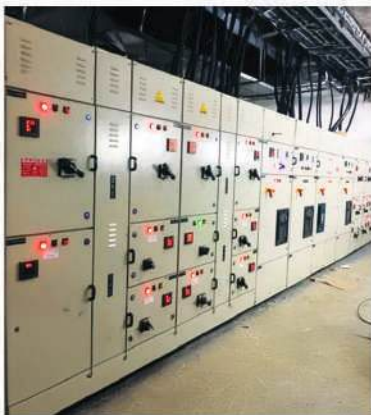
Power Control Center (PCC)
