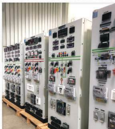
Relay Control Panels
