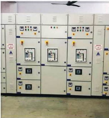
DG Load Management Panels
