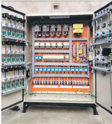
A.C. Drive Panels (VFD)
