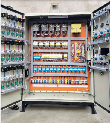
A.C. Drive Panels (VFD)
