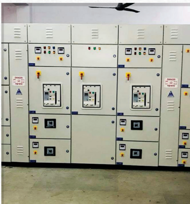
DG Load Management Panels
