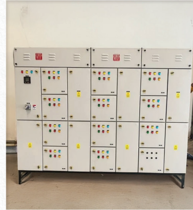
Motor Control Center (MCC)
