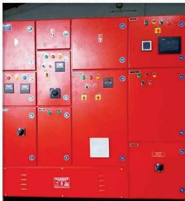
Fire Fighting Panels
