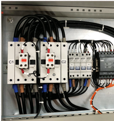
Auto Transfer Switch (ATS)
