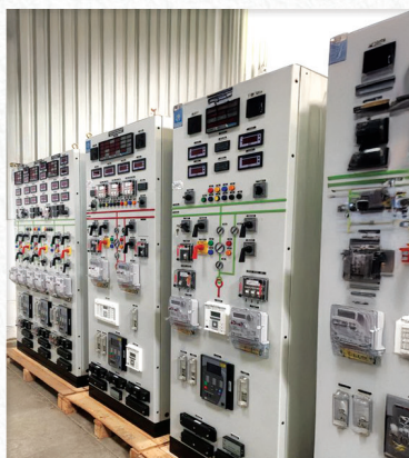
Relay Control Panels
