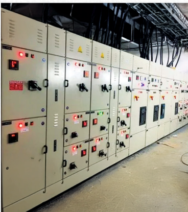
Power Control Center (PCC)
